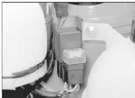
3.7a Headlamp washer relay and fuse
