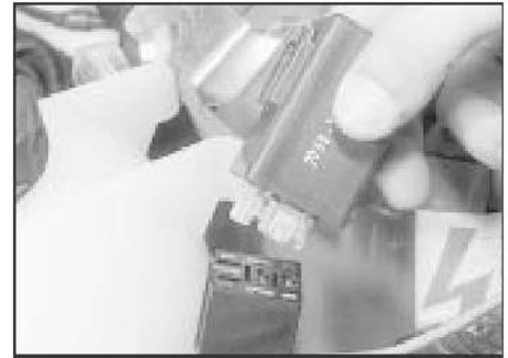
12.36b Unplugging the control relay
