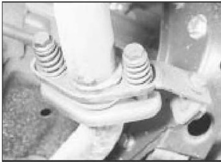
27.4a Exhaust system flexible joint
