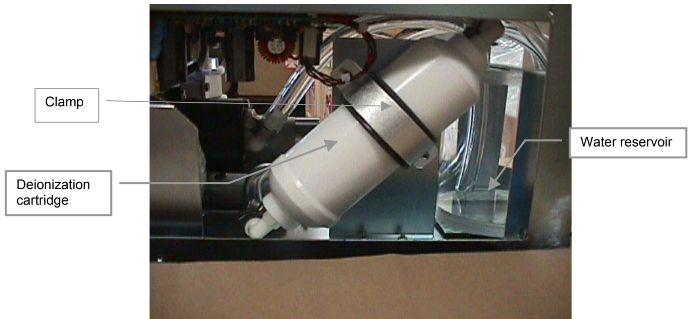
Figure 5-1. Cooling System in the Power Supply
