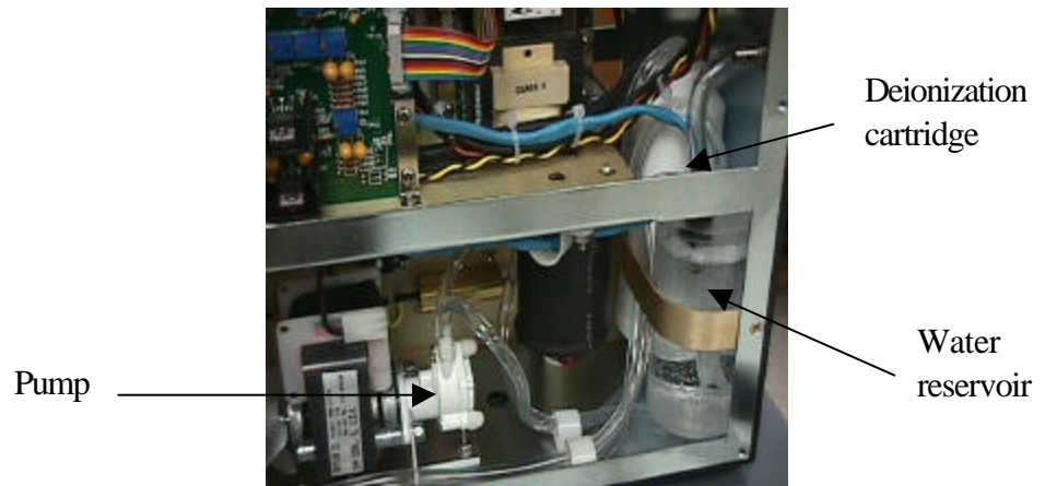
Figure 6-1. Cooling System in the Power Supply
