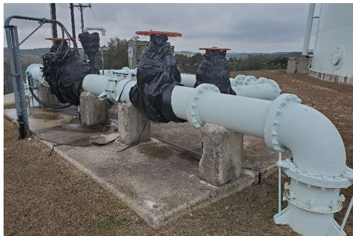
Figure 4: Temporarily Insulated Valves at Shields PS
