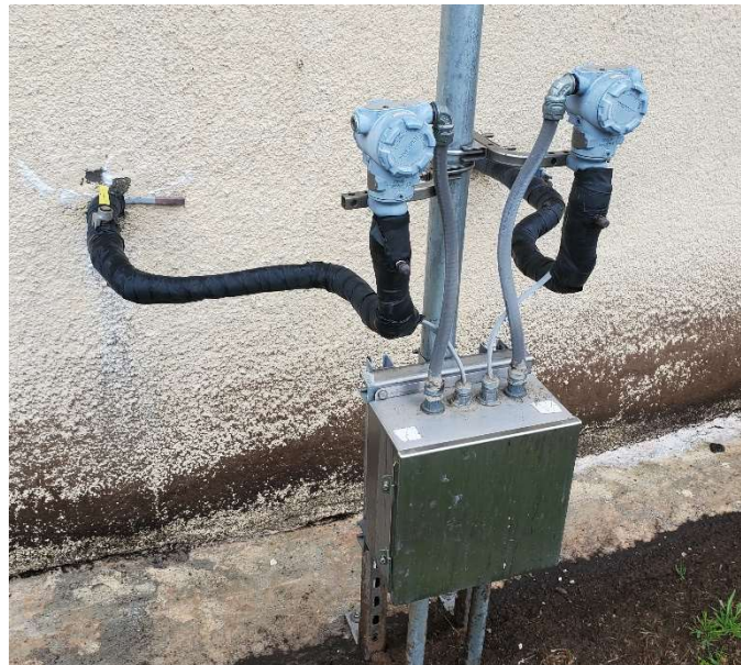
Figure 9: Pressure Style Level Transmitters Heat Traced and Insulated at Winwood GST
