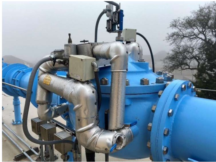
Figure 7: Heat Traced Control Pipe on PRV at Montana Pass PS
