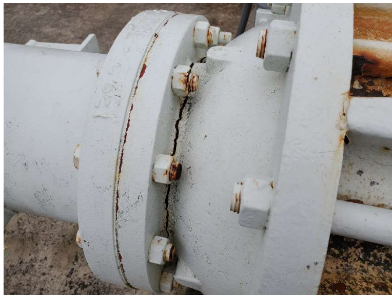
Figure 8: Cracked Valve Body at Winwood Pump Station
