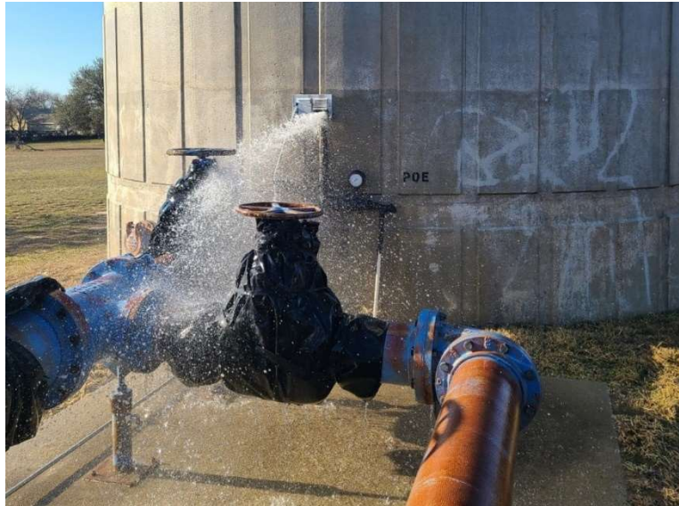
Figure 6: Broken Instrument, Pipe Leak & Insulated Valve
