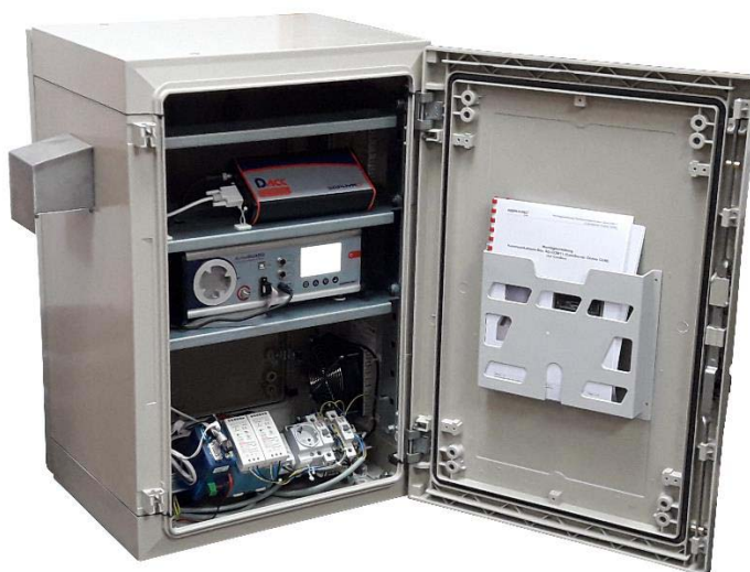
Figure 62: Example of remote monitoring station
