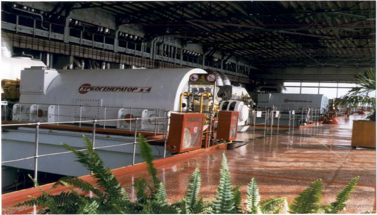
BN-600 turbine hall.
