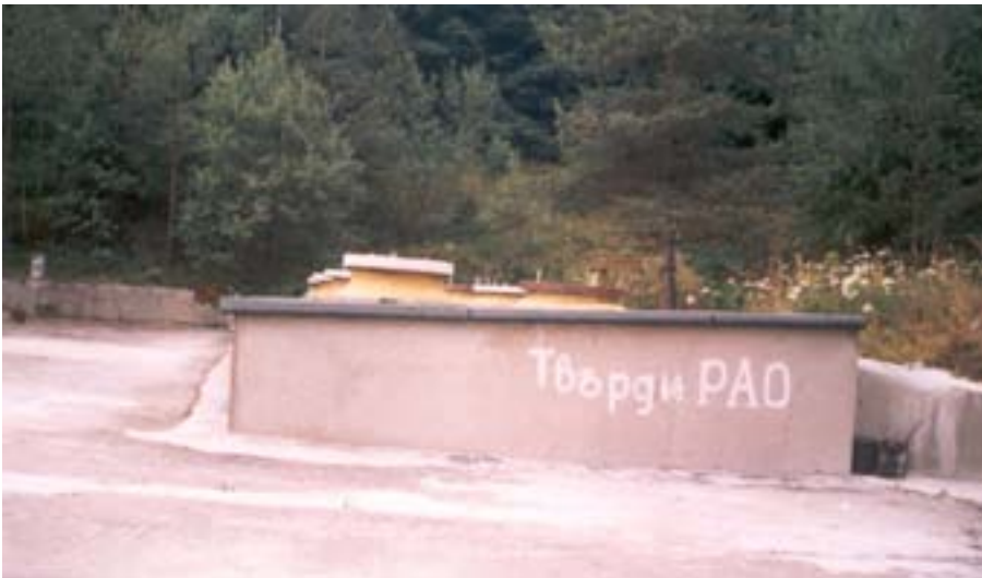
FIG. 12. Disposal vault for solid waste after improvement.
