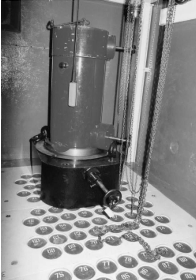
FIG. 18. Small storage facility for vitrified LILW (Slovakia).
