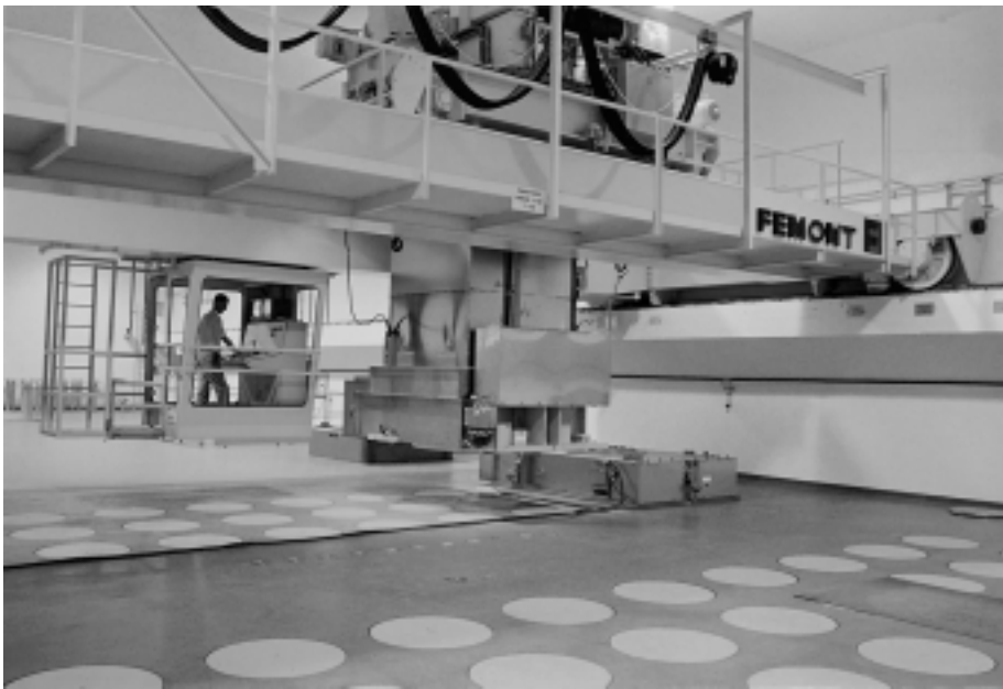
FIG. 26. Charging machine on top of the interim storage cell for vitrified HLW canisters (France).
