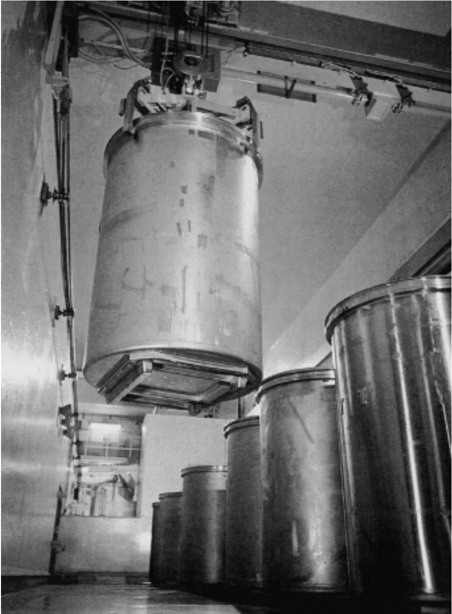
FIG. 5. 1500 L stainless steel container for cemented cladding hulls and end fittings (France).
