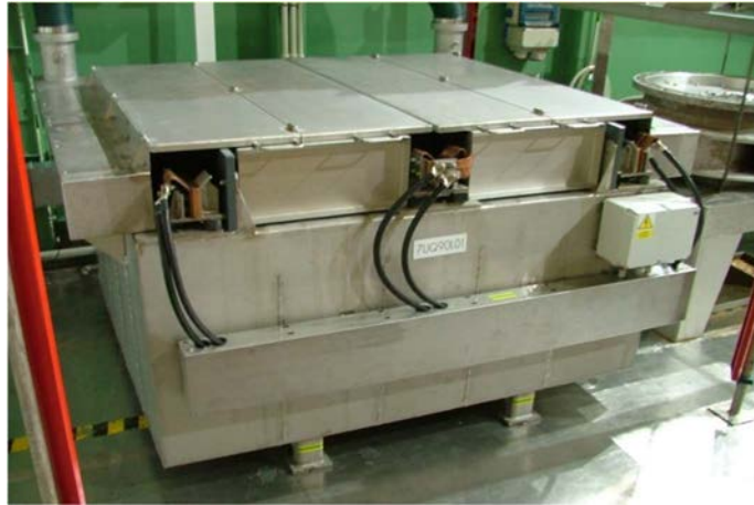
FIG. I-6. Electrochemical decontamination bath CEZ a.s., Dukovany NPP.
