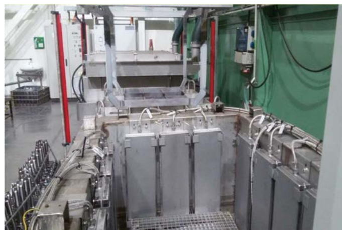
FIG. I-5. . Ultrasonic decontamination bath with transducers CEZ a.s., Dukovany NPP.
