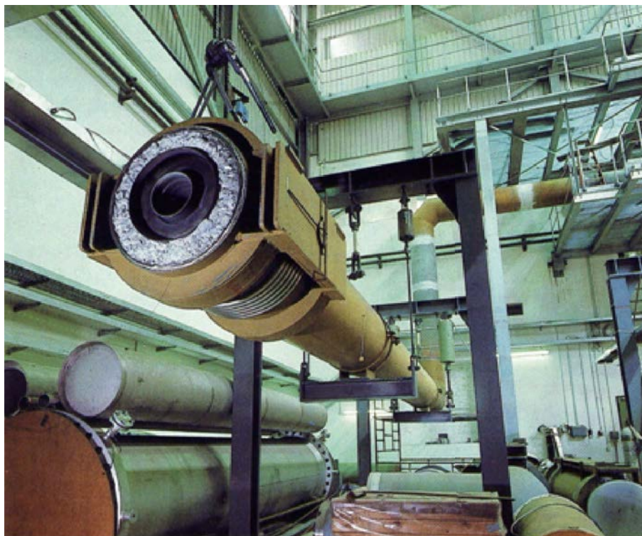
FIG. 102. Hot gas duct in the German KVK loop test facility [291, 292].
