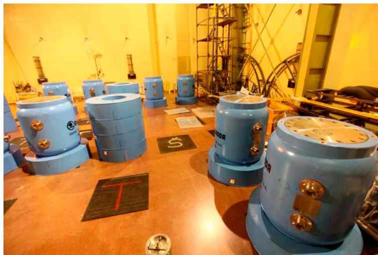
FIG. 1. Spent fuel containers.
