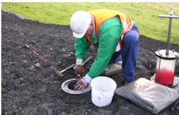
FIG. 4.4. Hand excavation of disturbed soil sample and measurement of in situ natural density using the balloon method. (Courtesy of Department Mining Remediation/Geotechnics, Wismut).
