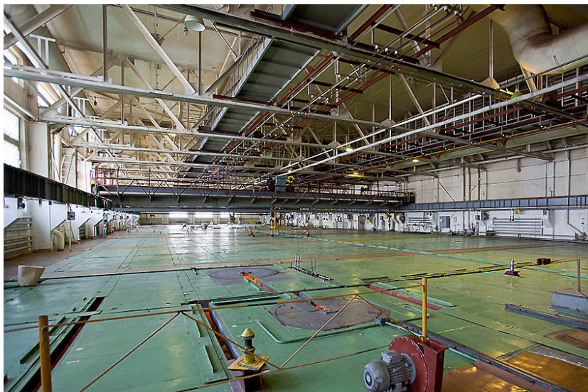
FIG. 9. General view of the SNF pool at FSUE Mayak PA.
