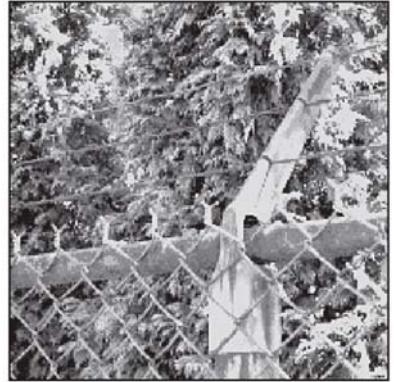
Figure 5: Rust near the transmitter
