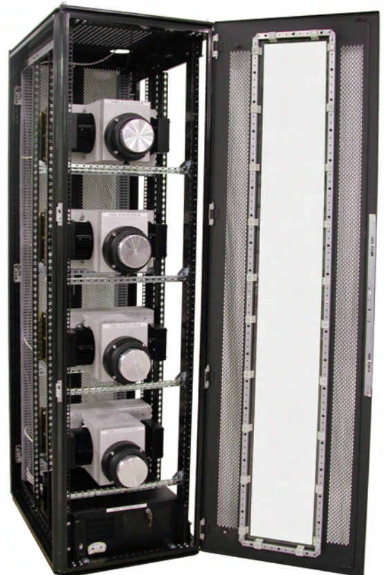
Figure 2. IDMs mounted in cabinet.
