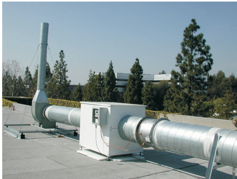
Pic.2 : PET Stack Monitor with Gas Flow Sensor in front. The transmitter for the Gas Flow Sensor is mounted at the PET Stack Monitor.
