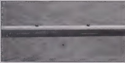
Figure 21.40 — Element splice uses a 1 foot length of 0.75 inch tubing inserted into the 0.875 inch sections to join them together. Self-tapping sheet-metal screws are used in this photo, but aluminum pop rivets or machine screws with washers and nuts can be used.
