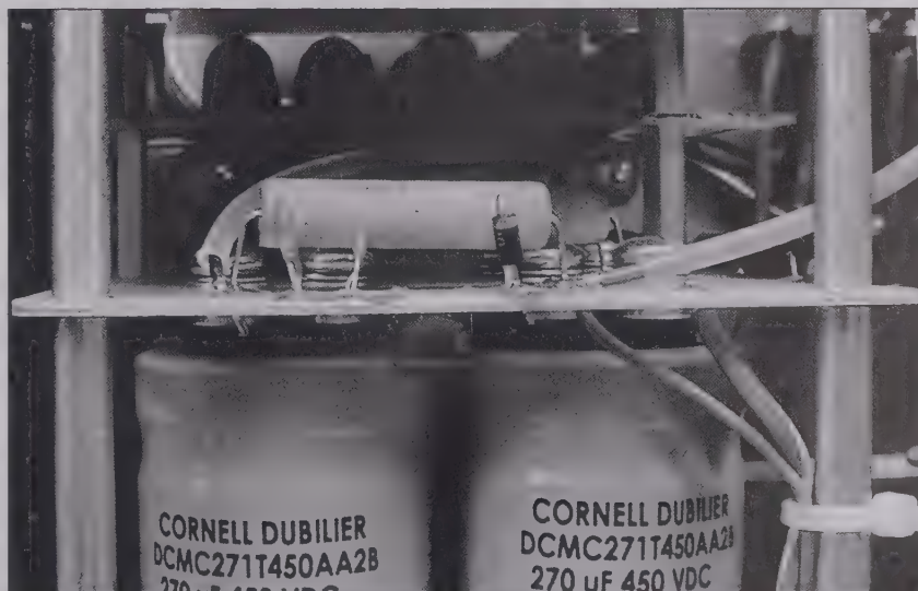
Figure 7.44 — Example of the filter capacitor/bleeder resistor installation in a high voltage power supply.
