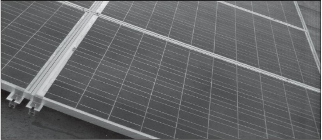
Figure 2.9 — Solar power receiving antenna. The more panels, the more aperture, the more gain, and thus the more power recovered.
